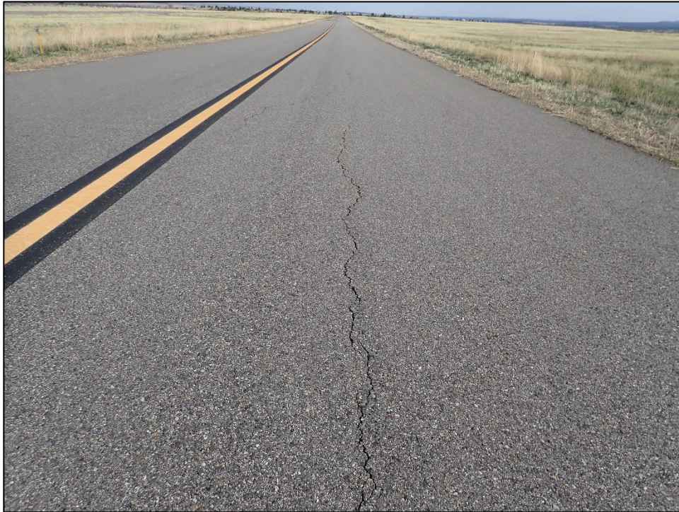
TW-04-11: L&T Cracking
