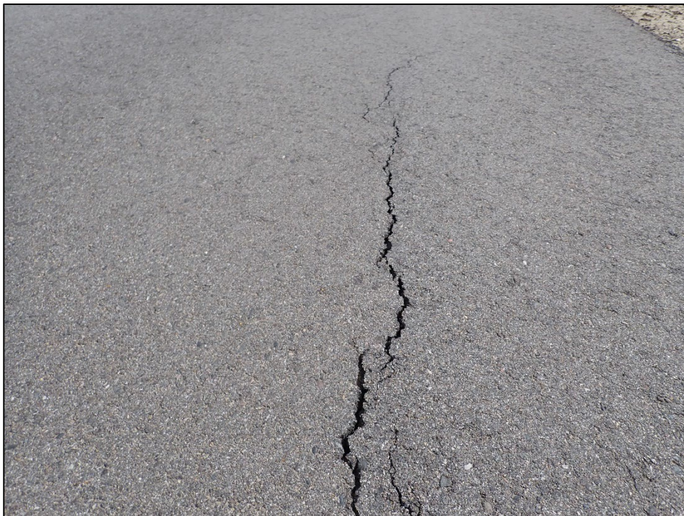
TW-07-01: L&T Cracking
