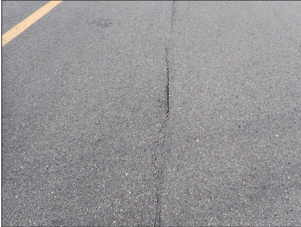
AP-01-01: L&T Cracking
