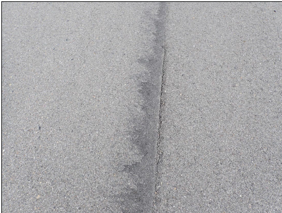
RW07-01-34: L&T Cracking
